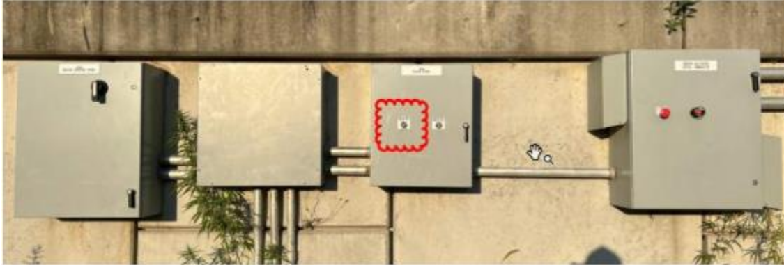
Pull up float switch controlling motor inside waterfall fountain pump station.
