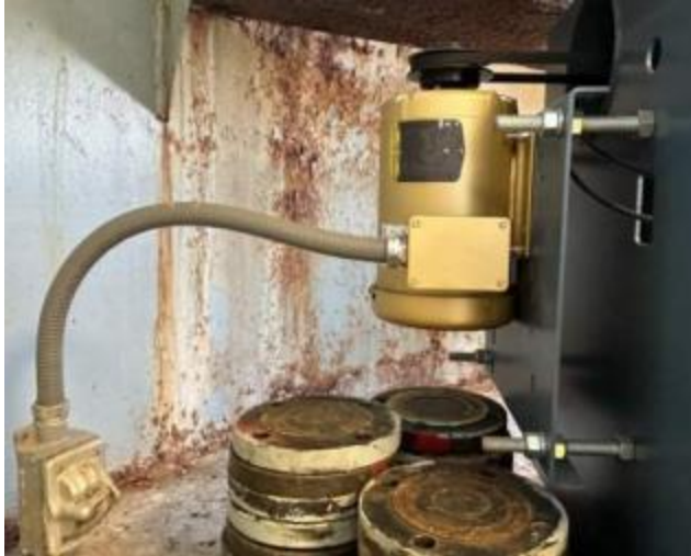
Blow out heaters of dust (2 locations)
